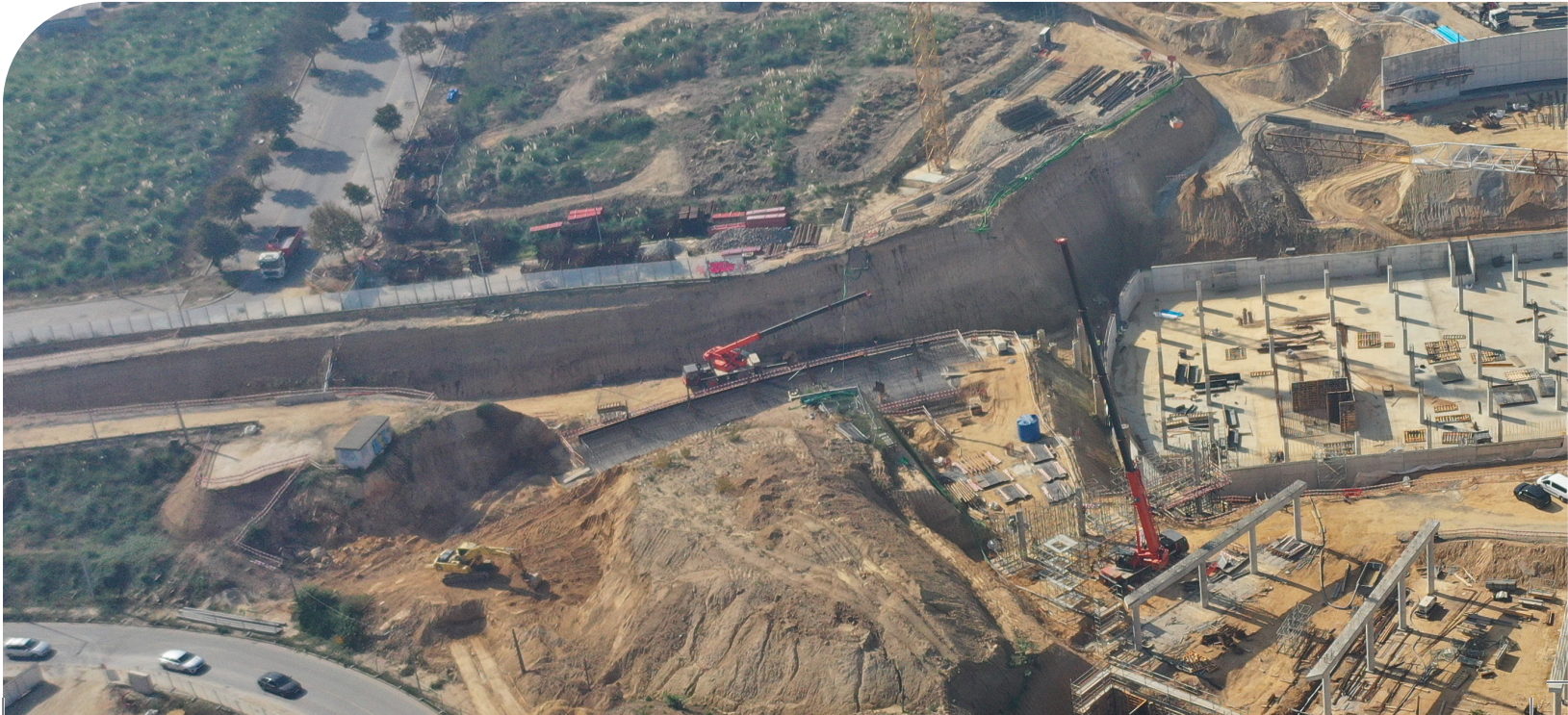
New Ruby Line Metro Station, Porto – Portugal
