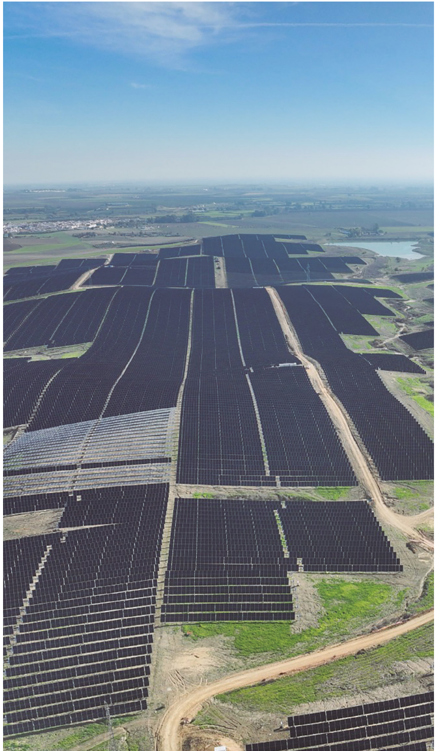
Guillena photovoltaic park (Seville, Spain)
