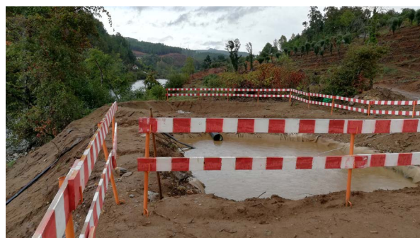
Water settling basin.
