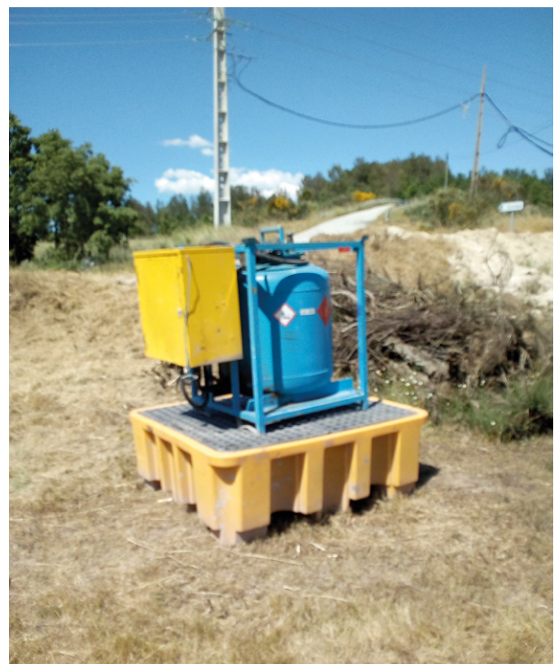
Discharge containment tank.
