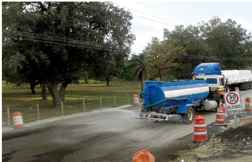
Watering of trucks, use of tarpaulins during material transportation and speed limit measures.
