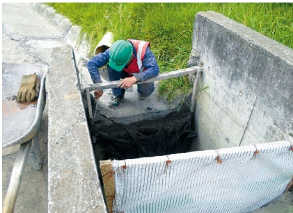
Desander of the waters coming from the rain and runoff
