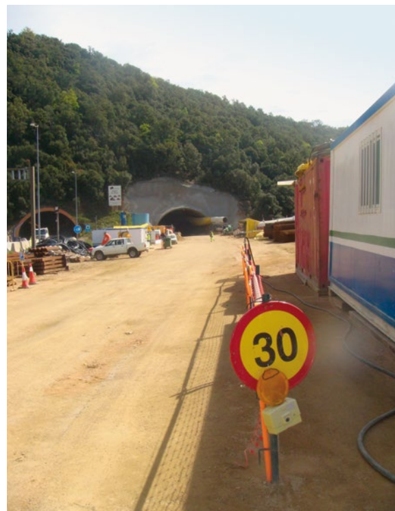
● A suitable control of vehicles' speed on site contributes to the minimisation of dust emissions and noise, both aspects being intrinsic to these operations.
